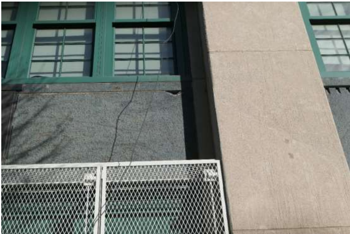
Photo M06 – Halfmoon crack and missing granite piece at South Façade.
