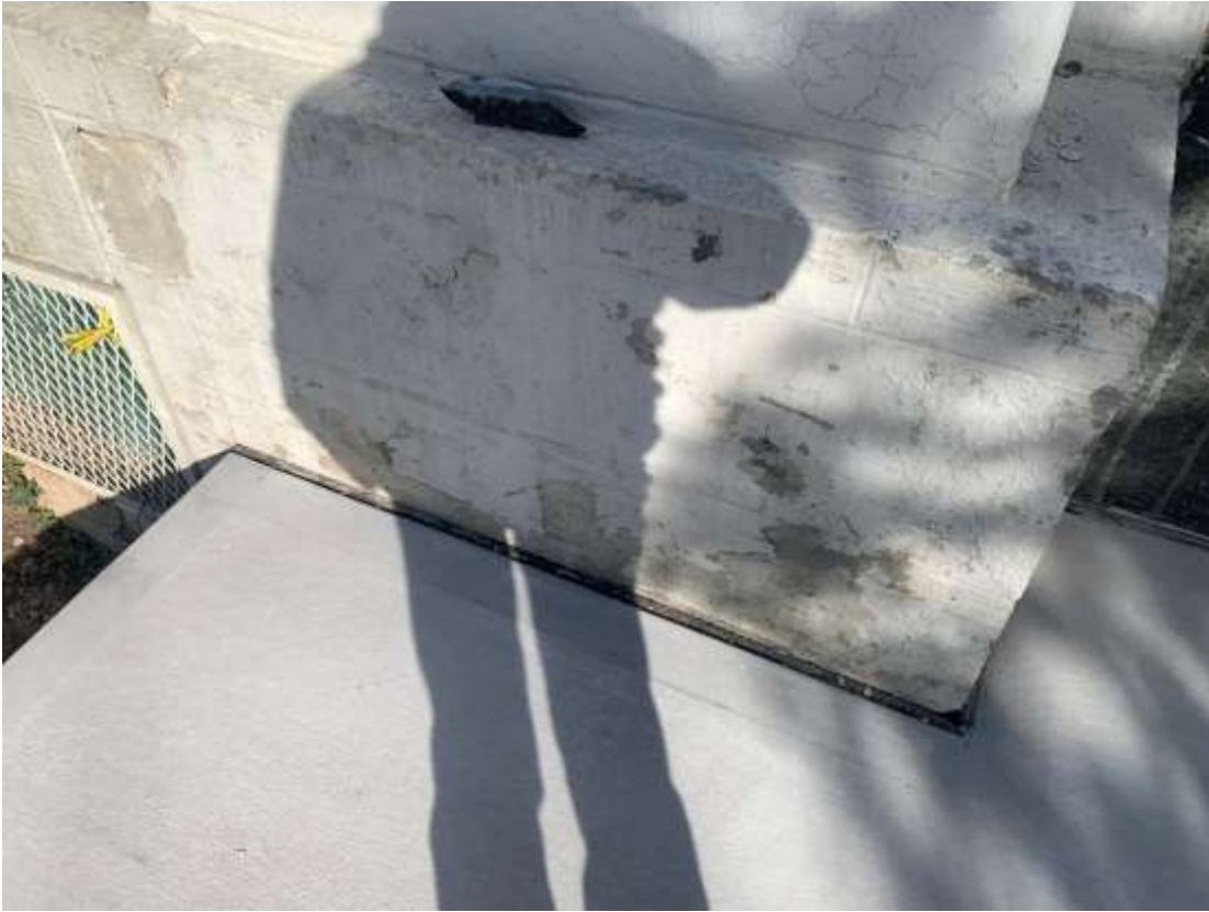
Photo M07 – Open joint at stairs landing at South entrance.
