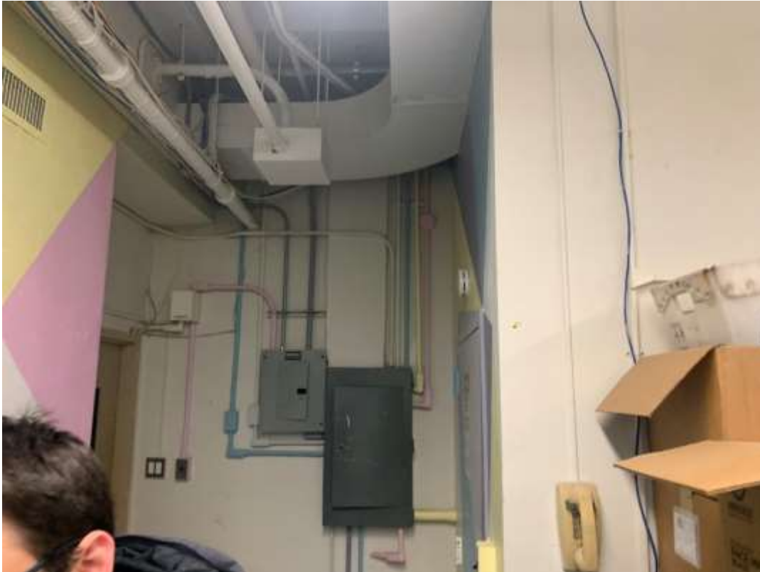
Photo A05 – View of electrical panels at room B2A.
