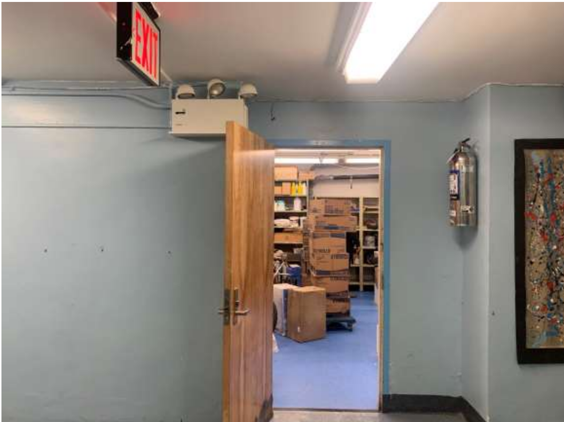
Photo A08 – View inside storage room B4 and damaged door.
