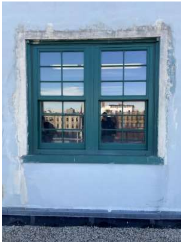
Photo M52– Damaged stucco in windows perimeter indicates water infiltration – North Bulkhead Façade.
