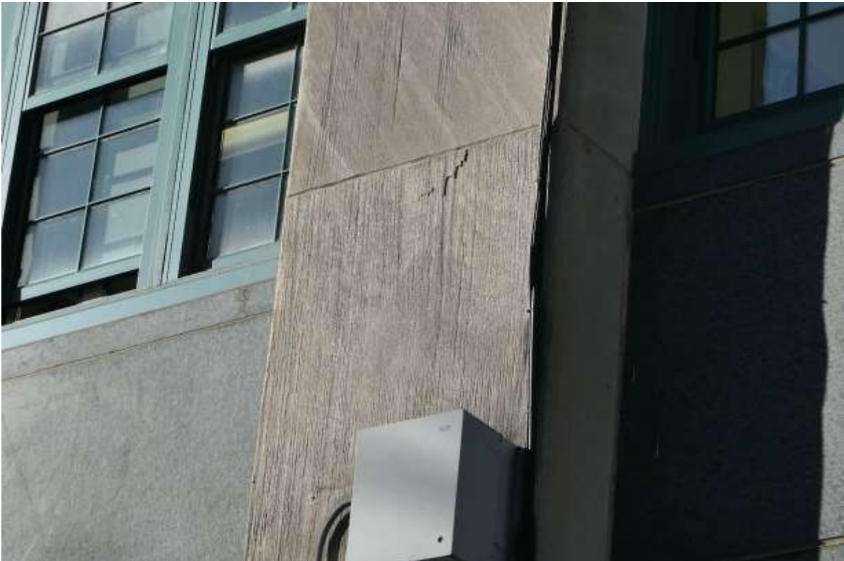
Photo M22 – Flake in limestone – East Façade.
