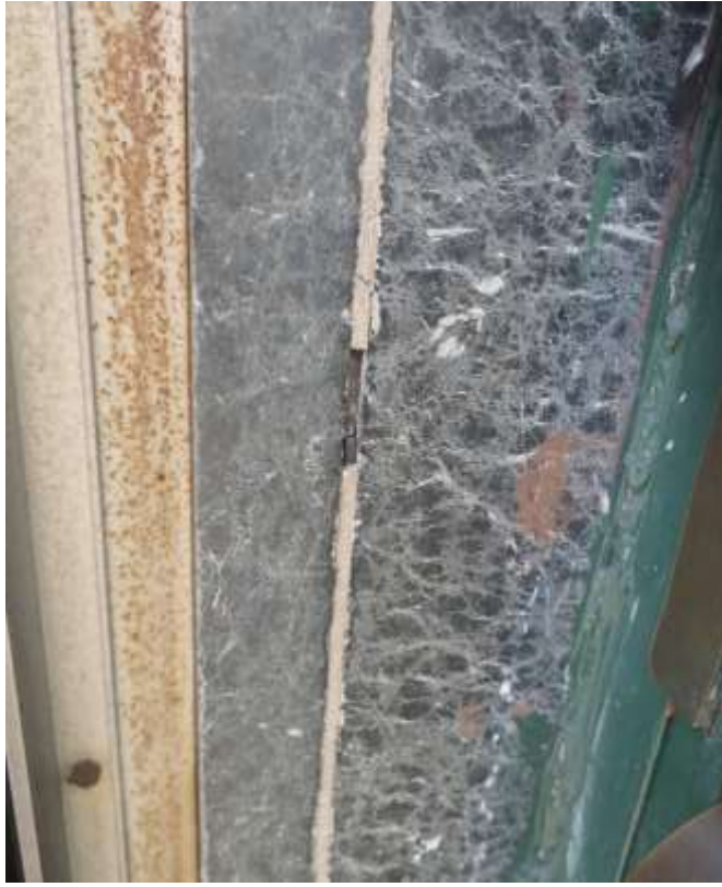
Photo M25 – Loose missing grout at stone.
