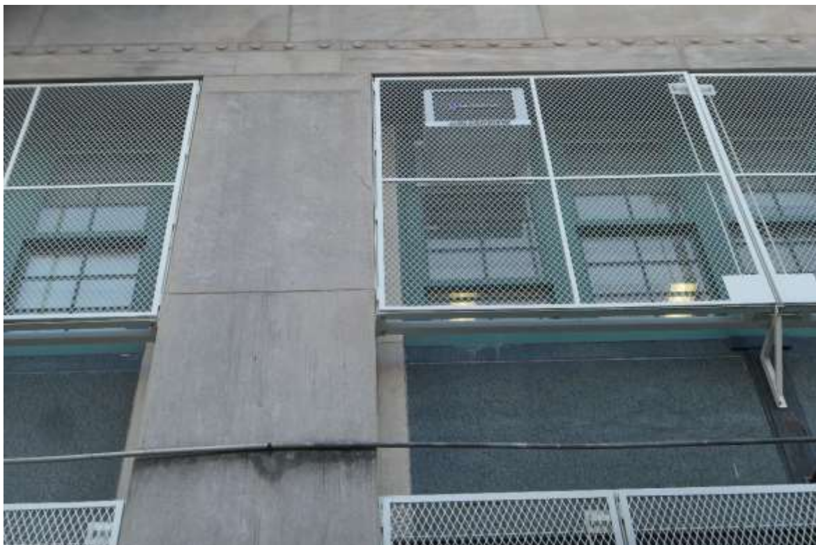
Photo M30 – Flake in limestone at North Façade.
