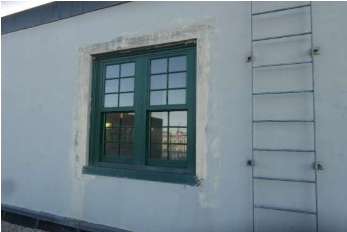
Photo M49 – Damaged stucco in windows perimeter indicates water infiltration, roof ladder is in good condition – North Bulkhead Façade.
