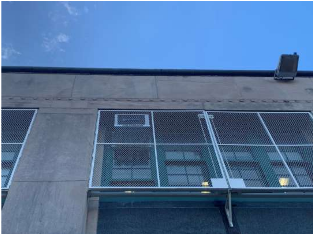
Photo M32 – Crack in Limestone, window guards are in good condition – North Façade.
