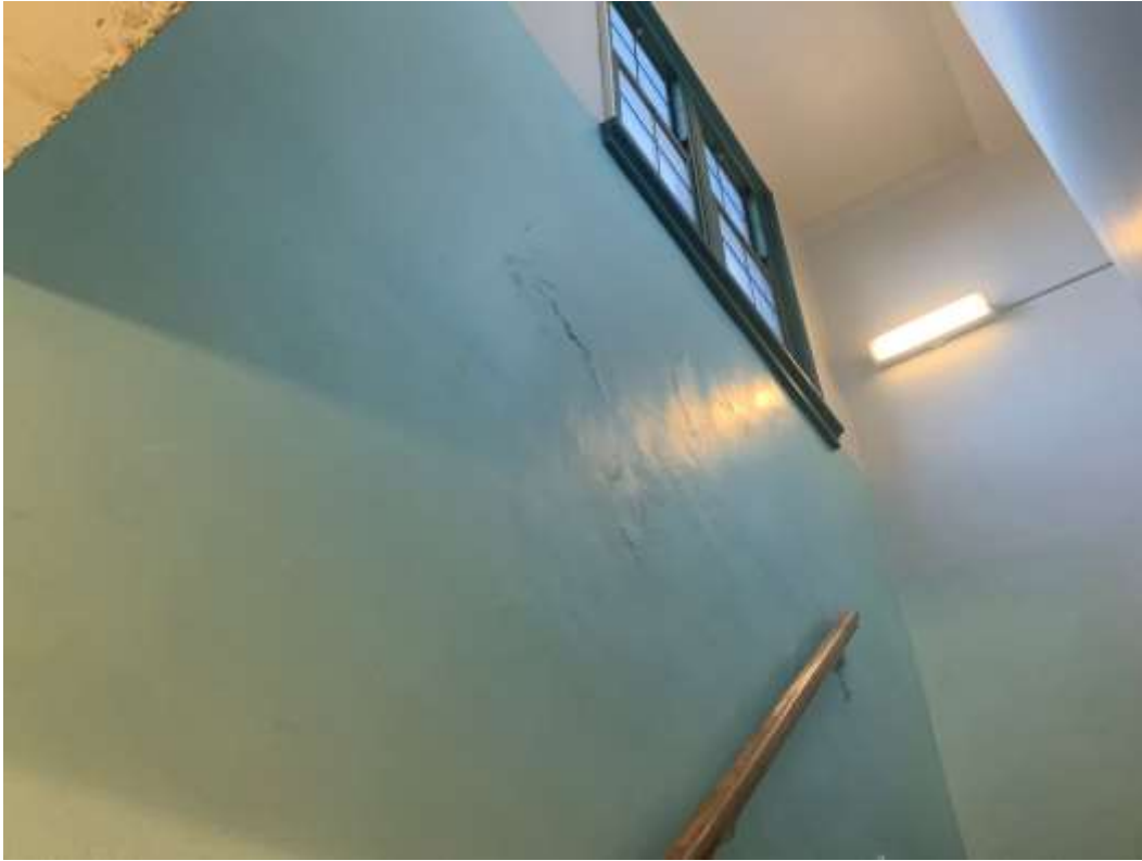
Photo A36 – Damaged interior plaster in bulkhead at wall in stair #2 area, indicates water infiltration.
