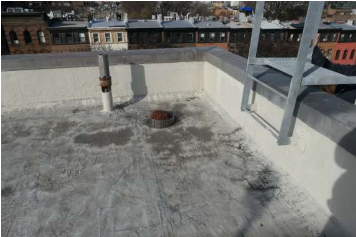
Photo P08 – Bulkhead parapet, roof drains and vents are in good condition.
