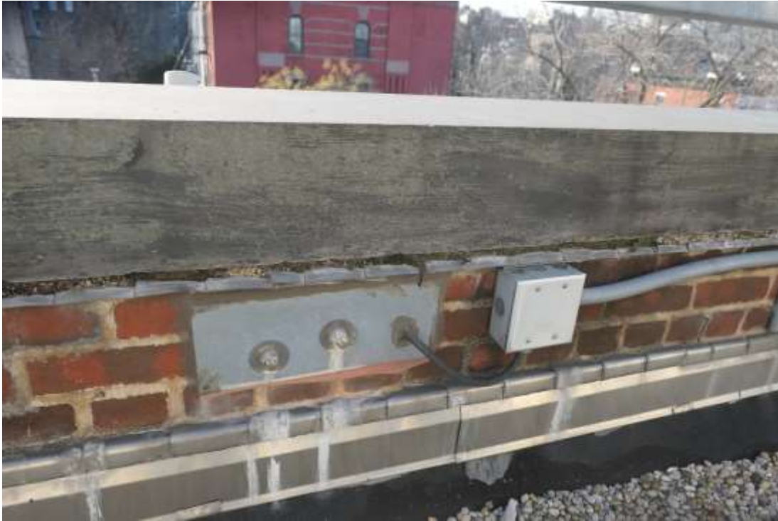
Photo P03 – Roof parapets are in overall good condition, there's some deteriorated brick joint mortar in some areas.
