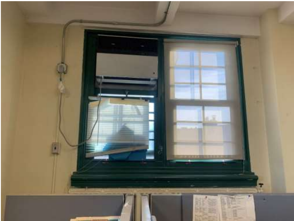
Photo A39 – Damaged interior plaster in bulkhead indicates water infiltration.
