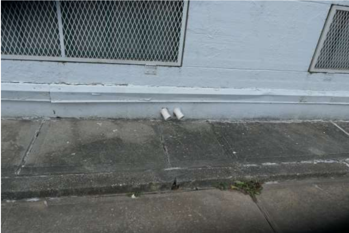
Photo S11 – Sidewalk at North façade next to parking driveway is in fair condition.
