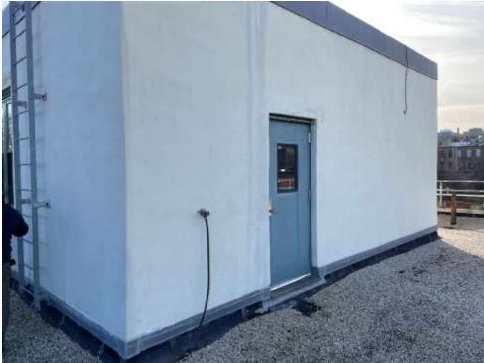
Photo M48 – Damaged stucco in bulkhead exterior door indicates water infiltration – West Bulkhead Façade.
