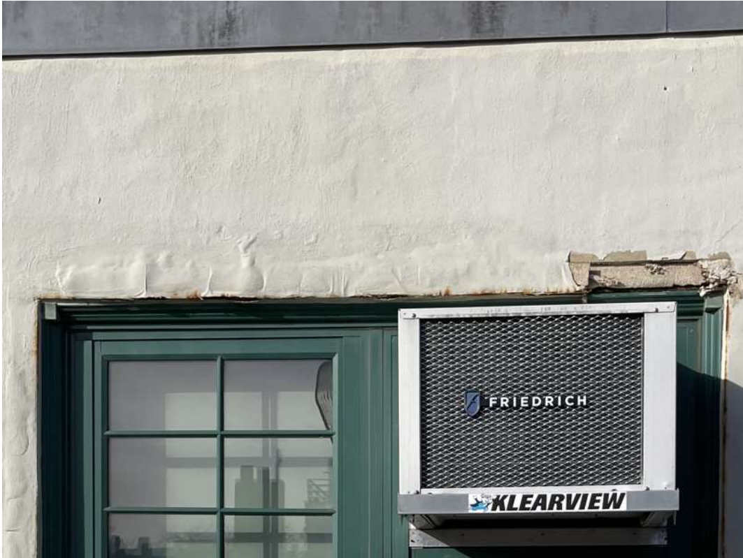
Photo M55 – Detail of damaged stucco and missing stucco in window lintel indicates the source of water infiltration – East Bulkhead Façade.
