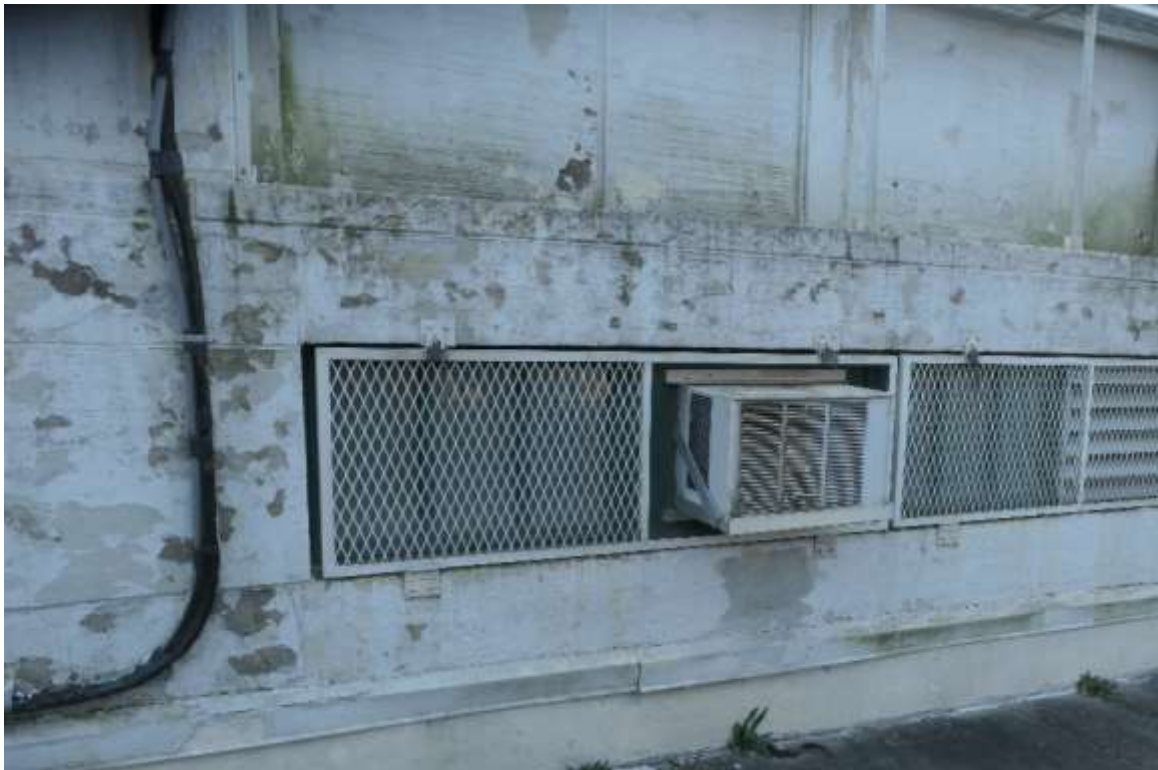
Photo M34 – Peeling paint – North Façade.
