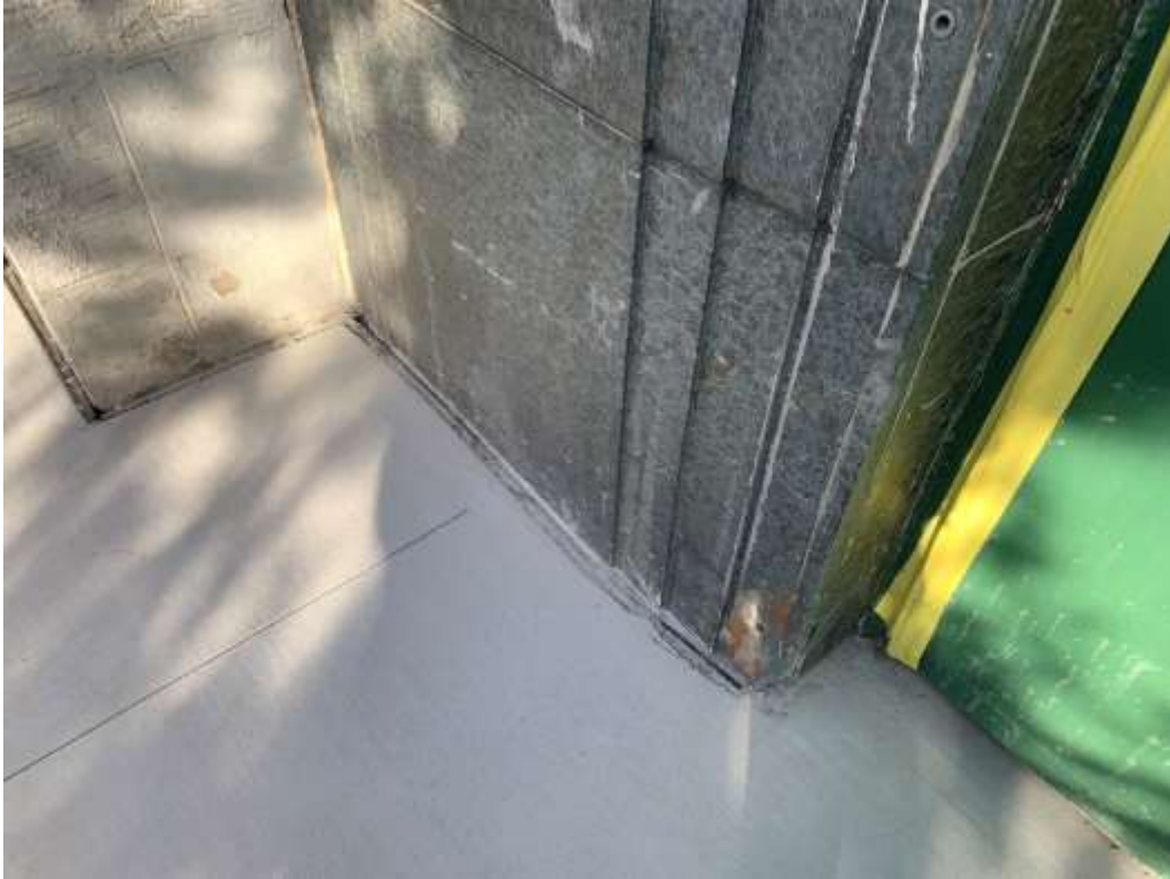
Photo M09 – Open joint between new landing and existing building's foundation at South entrance
