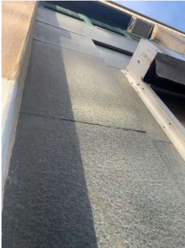
Photo M23 – Cracks at granite panels, East Façade.
