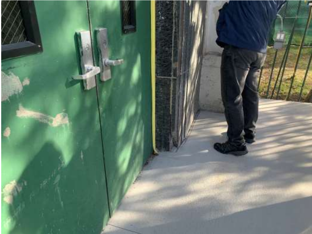
Photo M11– Missing stone and deteriorated mortar joint at Main Entrance.
