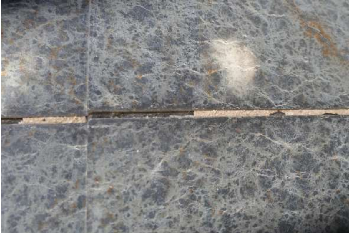
Photo M17 – Deteriorated mortar joints and loose missing grout at stone.
