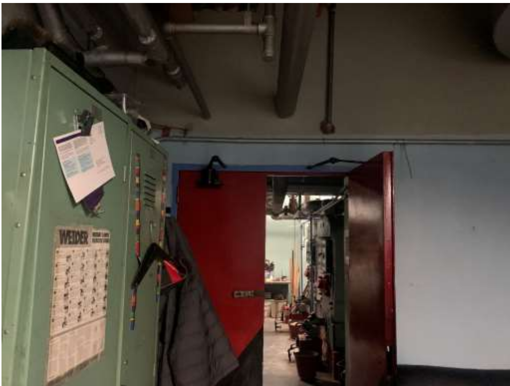
Photo A20 – Door at Boiler Room B7A towards Water Room B7B.
