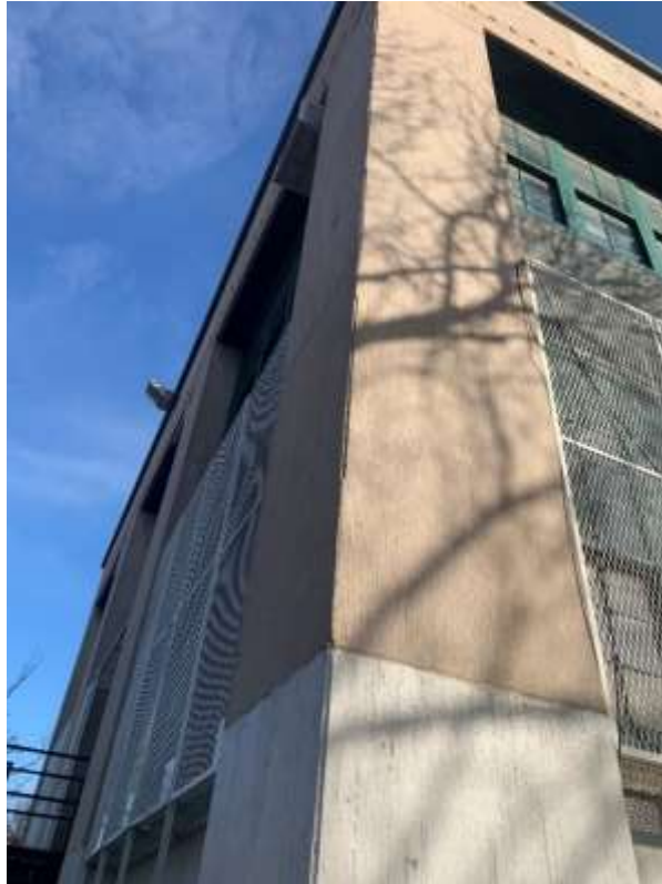
Photo M03 – Deteriorated joint grout at bottom area at Southwest corner.
