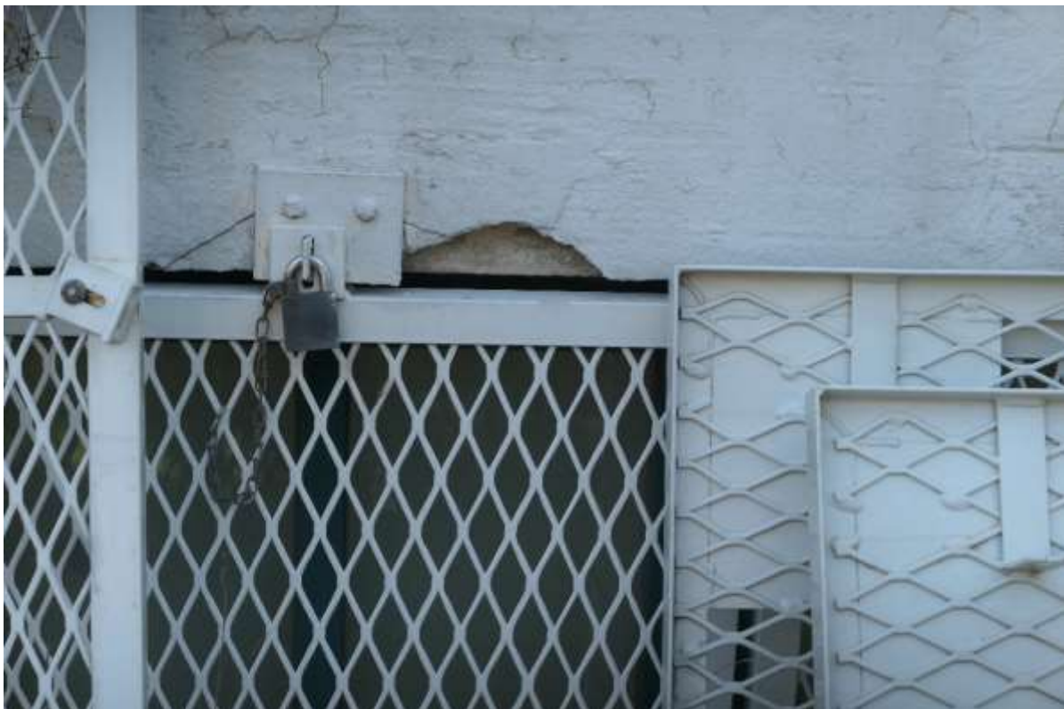
Photo M46 – Missing stone at West Facade.
