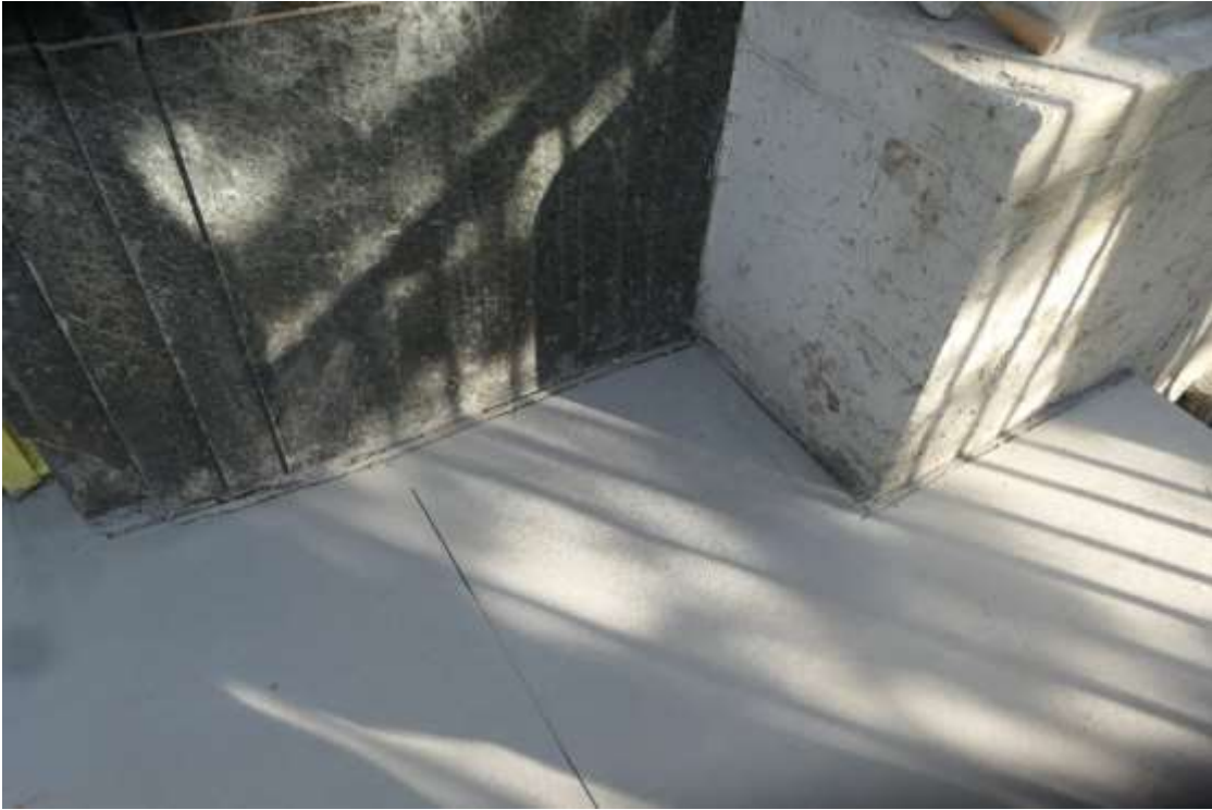
Photo M15 – Source of water infiltration at open joint between new landing and existing building's foundation at main entrance, south façade.
