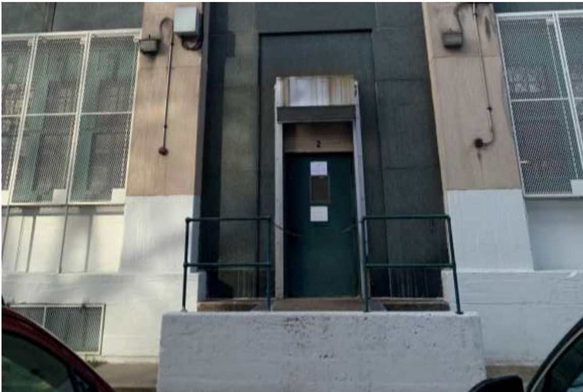
Photo S08 – Check walls and railing at East entry are in good condition.
