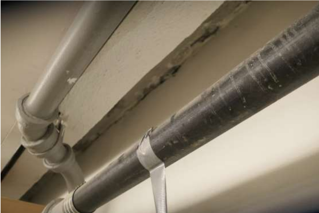
Photo A17 – Source of water infiltration is located at the ceiling line of Storage Room B4.
