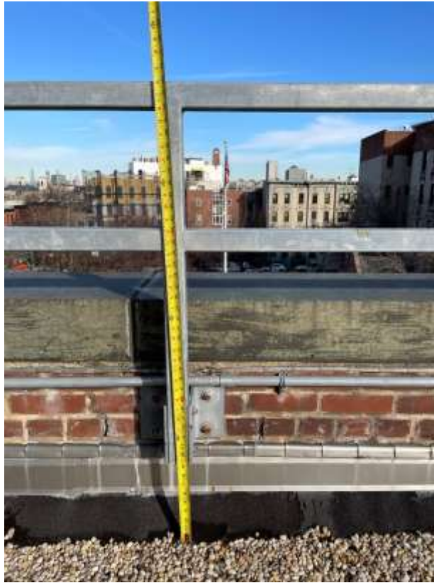
Photo P07 – Roof Barrier is up to code and in good condition.
