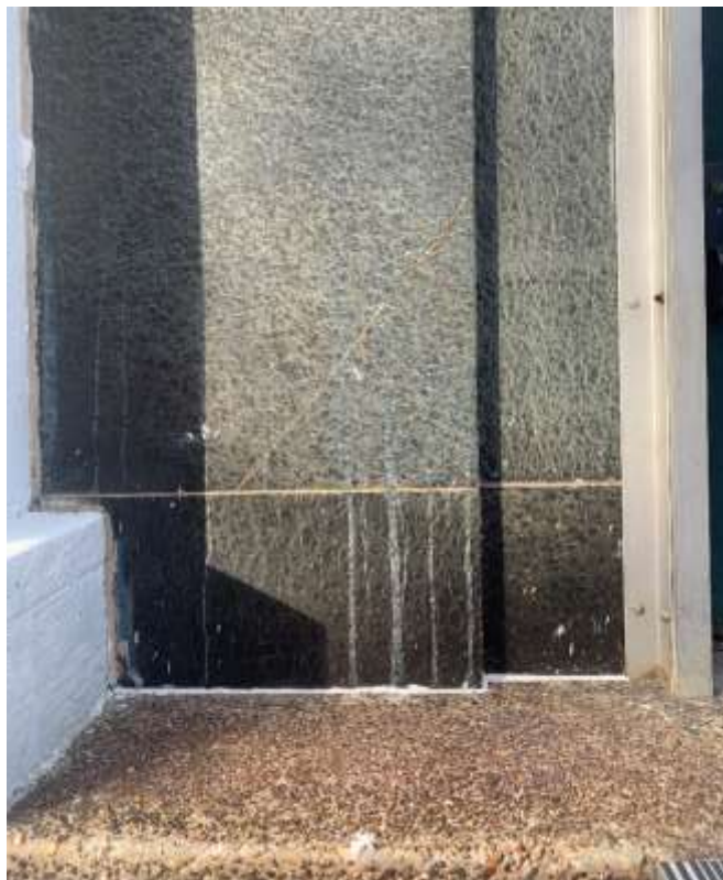
Photo M24 – Cracks at granite panels, East Façade.
