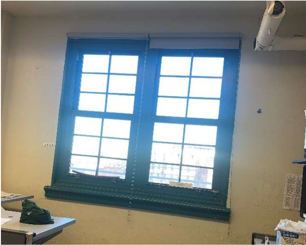
Photo A38 – Damaged interior plaster in bulkhead indicates water infiltration.
