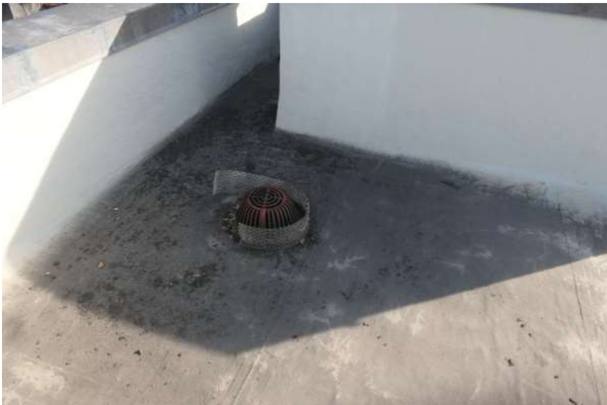
Photo R20 – Roof drains at Bulkhead roof are in good condition.
