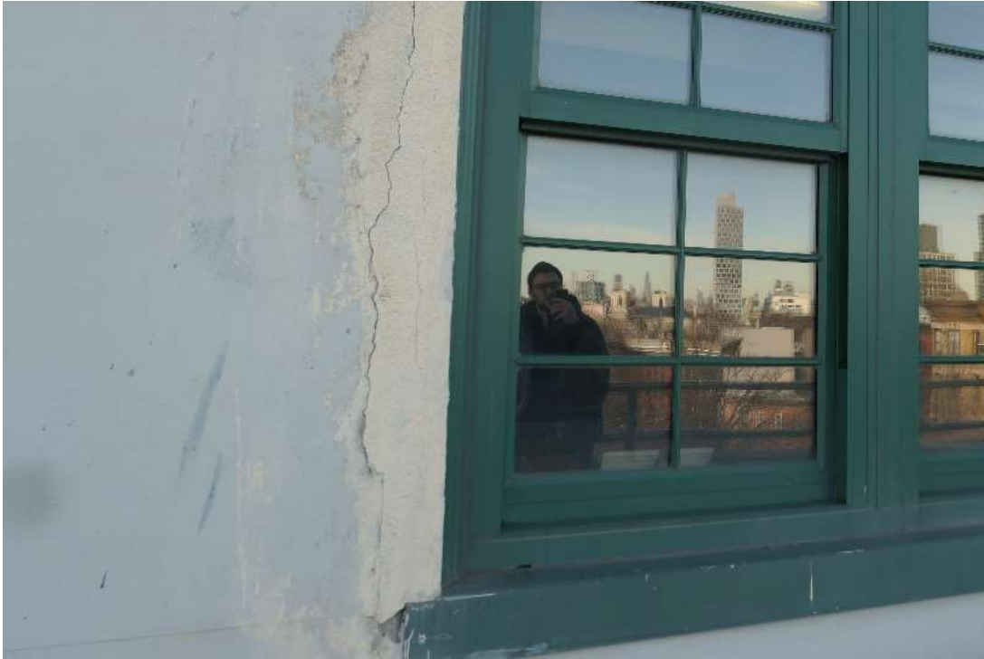
Photo M53 – Damaged stucco in windows perimeter indicates water infiltration – North Bulkhead Façade.
