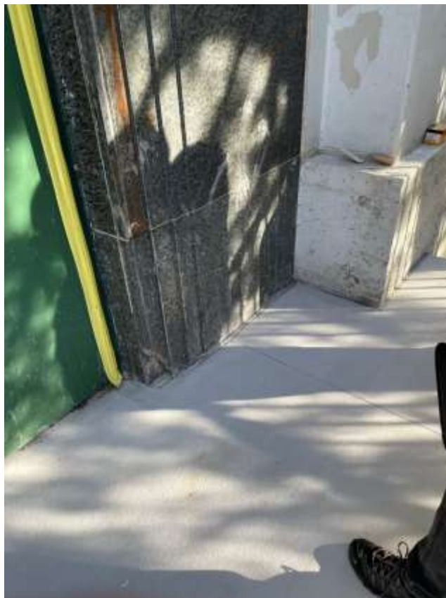
Photo M12 – Missing stone and deteriorated mortar joint at Main Entrance.
