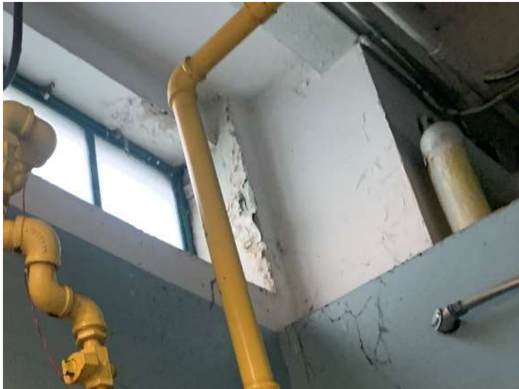
Photo A26 – Damage at plaster finish at Storage Room B3C
