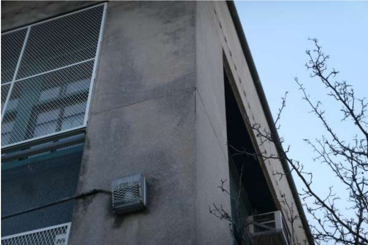
Photo M39 – Missing mortar at joints.
