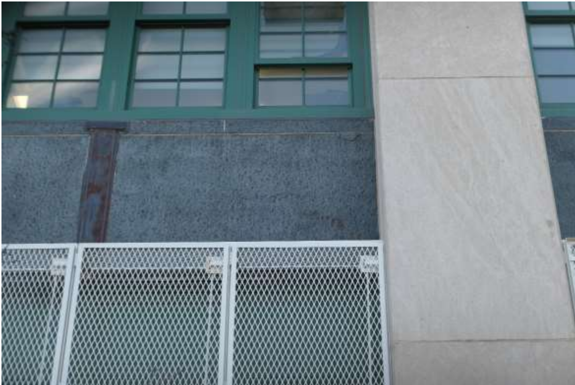
Photo M43 – Halfmoon crack in granite panel at West Façade.
