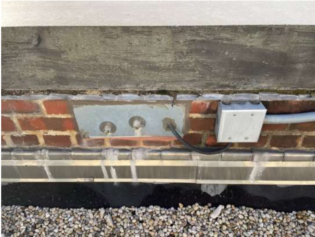
Photo P01 – Roof parapets are in overall good condition, there's some deteriorated brick joint mortar in some areas.
