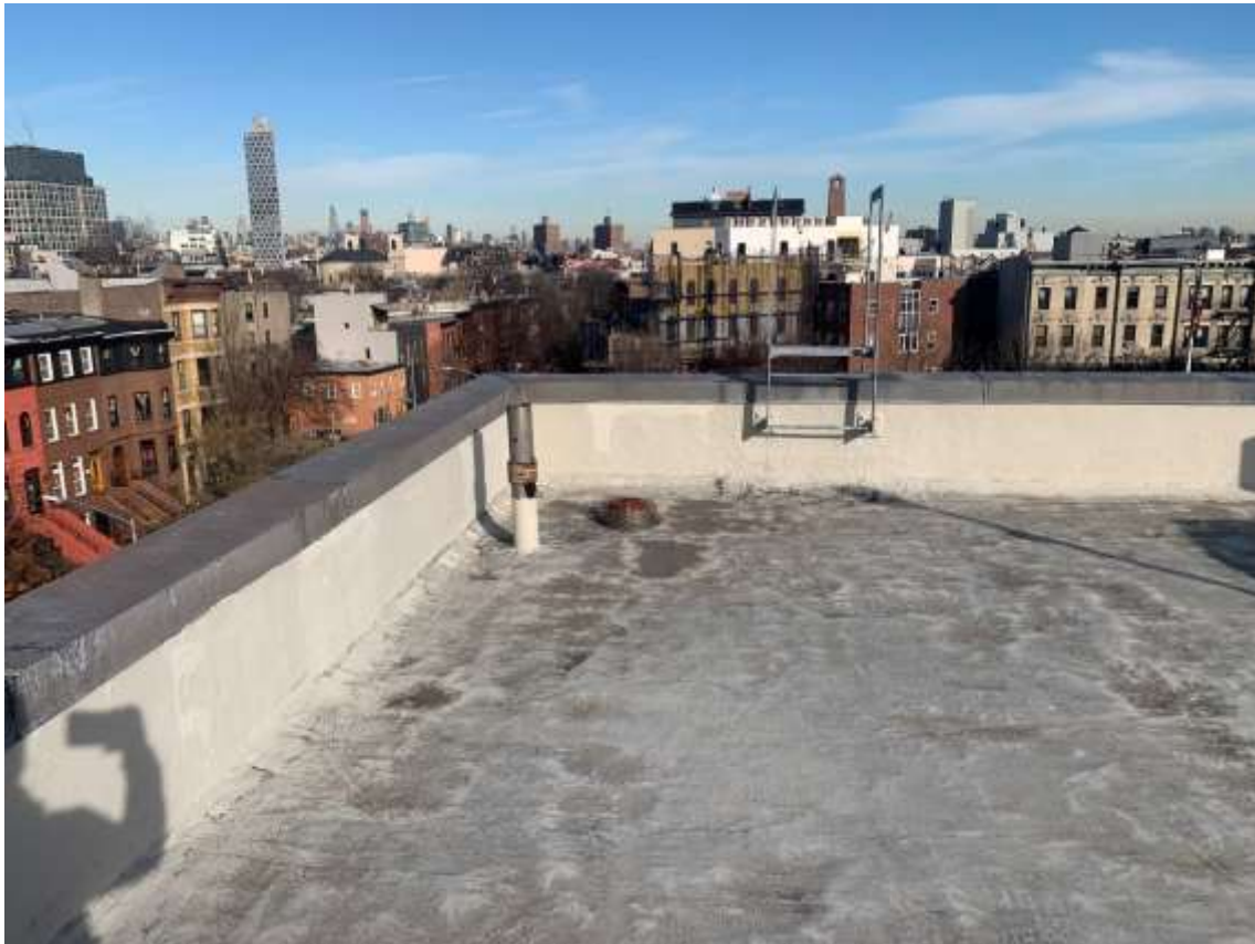
Photo R13 – View of bulkhead roof, roof ladder, vent and roof drain, facing North.
