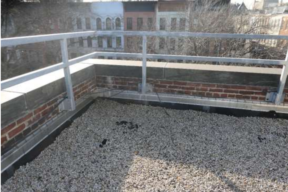
Photo P05 – Roof and roof barrier are in good condition, parapets shown some deteriorated brick joint mortar in some areas.
