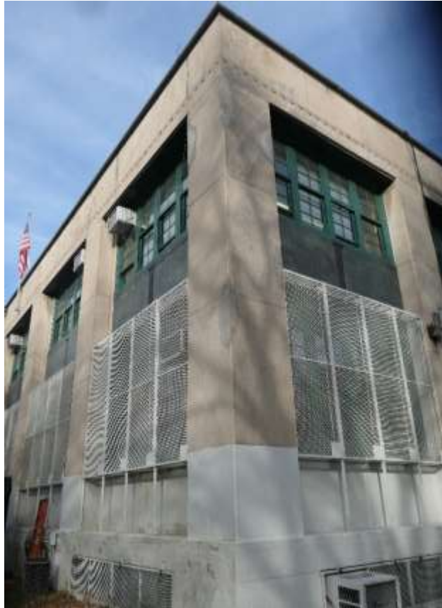
Photo M19 – Missing and deteriorated mortar joints at Southwest corner of the building.
