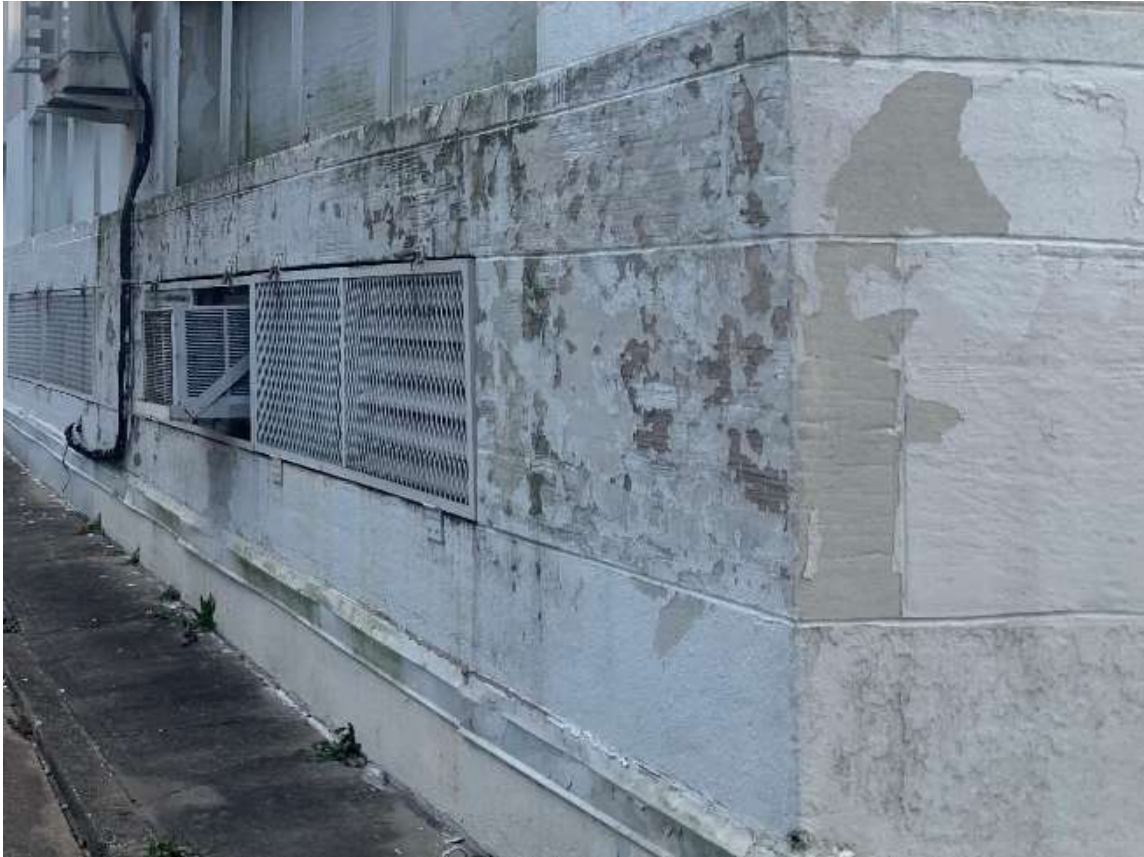
Photo M37 – Peeling paint – West and North Façade.
