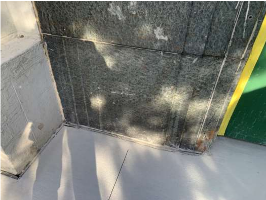
Photo M10 – Cracks and missing stone in granite at Main Entrance, South Elevation.
