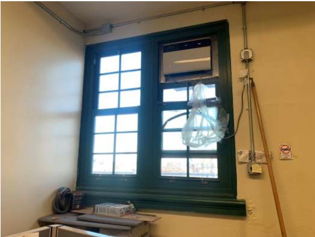
Photo A37 – Damaged interior plaster in bulkhead indicates water infiltration.
