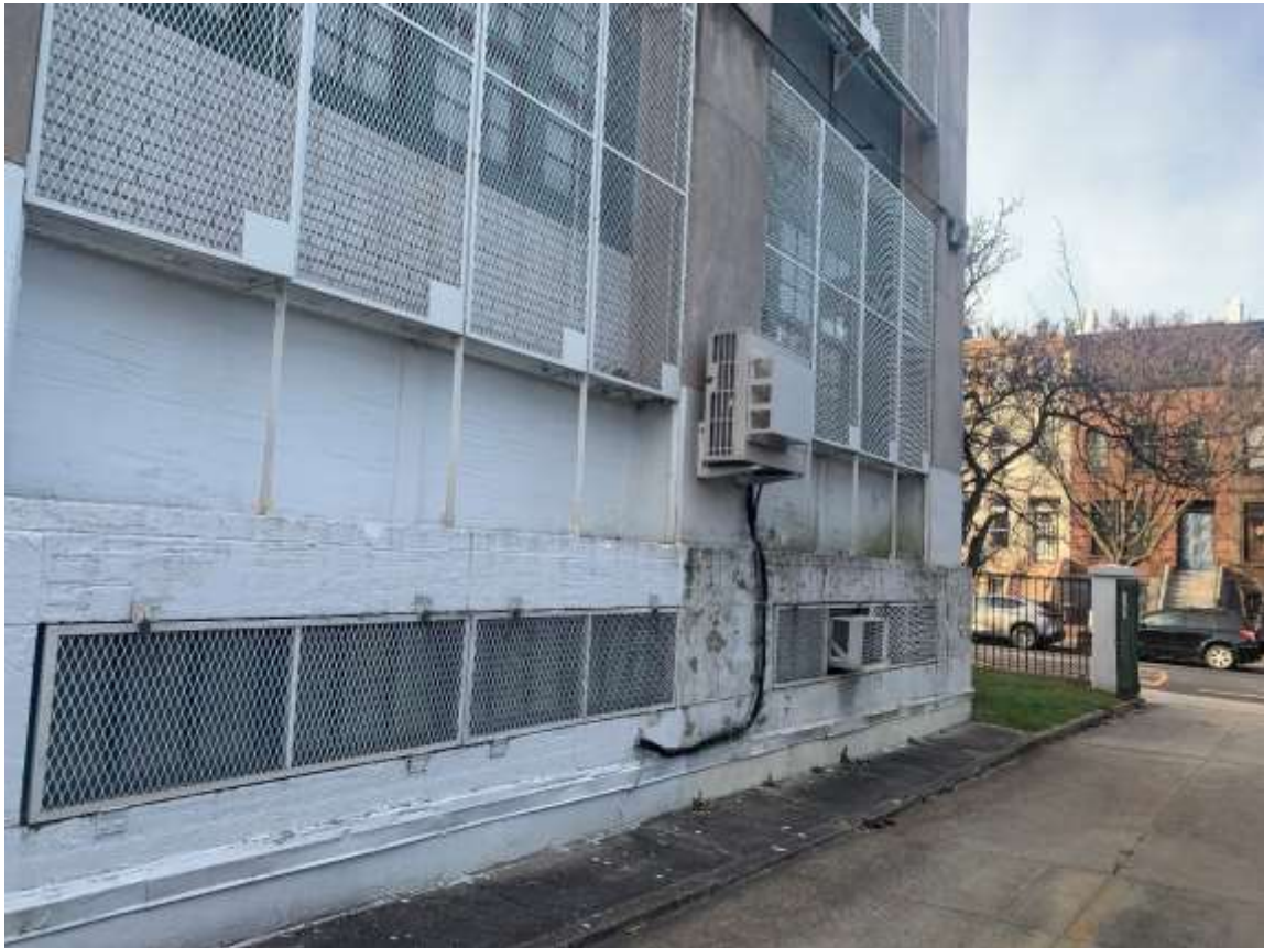
Photo M35 – Peeling paint area at North Façade.
