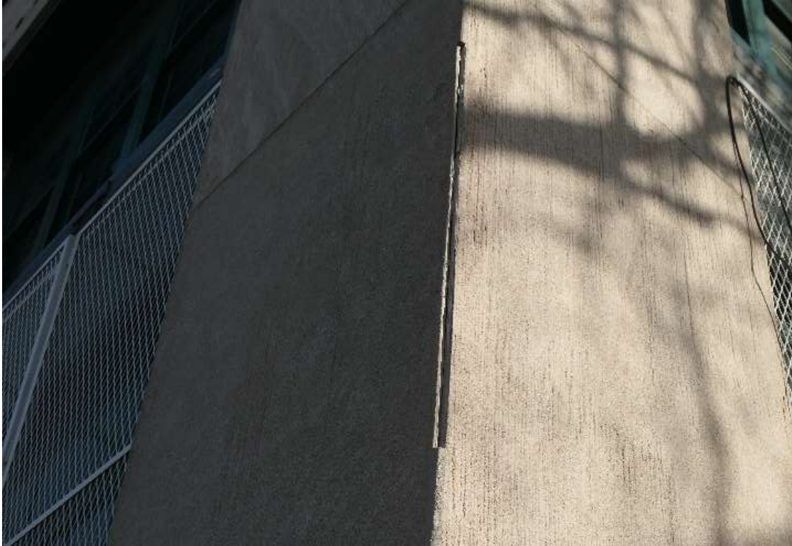
Photo M05 – Detail of deteriorated joint grout at Limestone.
