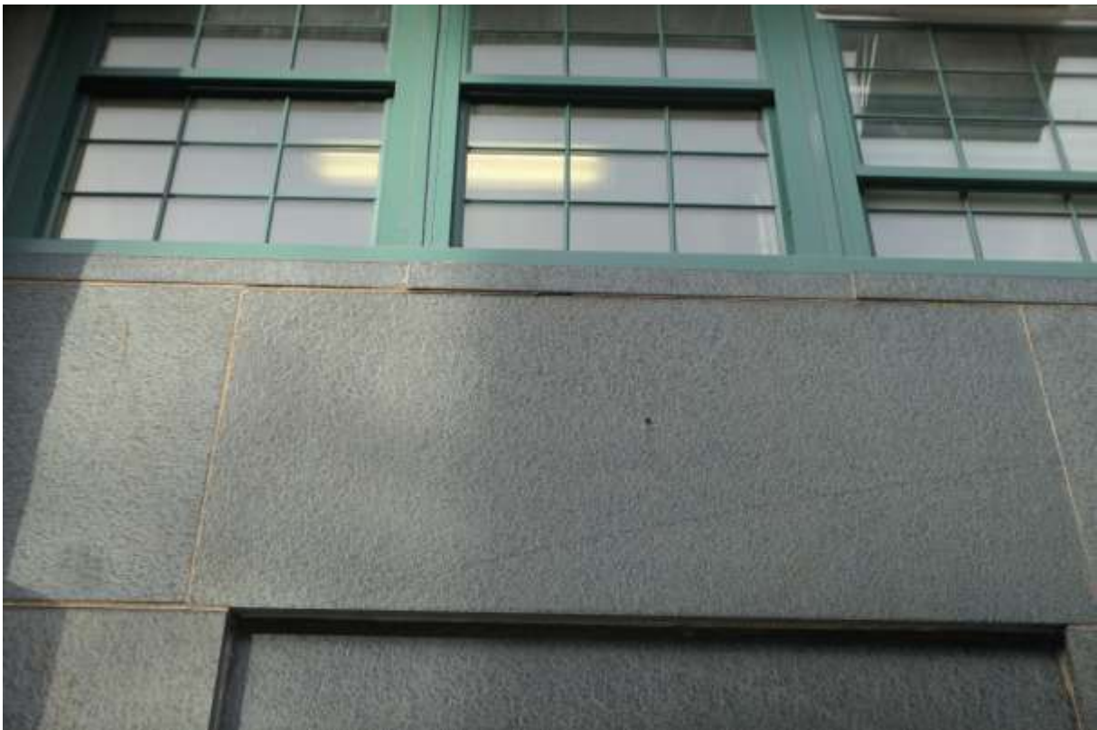
Photo M28 – Crack in granite above secondary entrance, East Façade.
