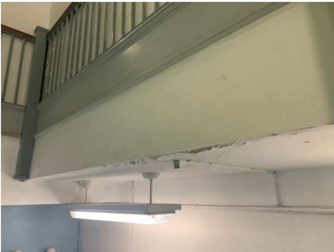
Photo A06 – Deteriorated ceiling at basement stair #2.
