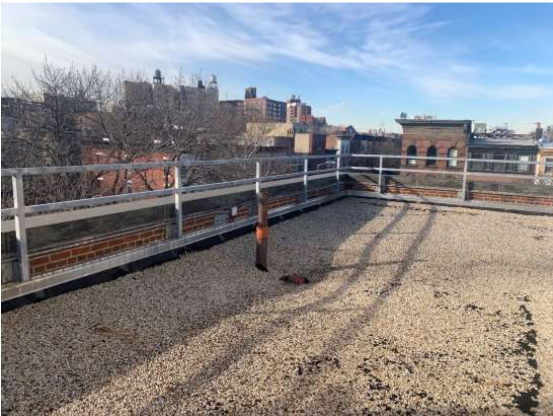
Photo P04 – Roof parapets are in overall good condition; roof is in good condition as well.
