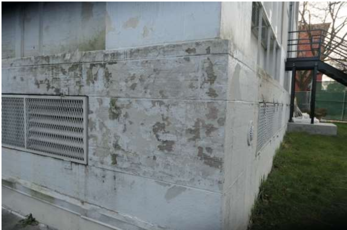
Photo M36 – Peeling paint – West and North Façade.
