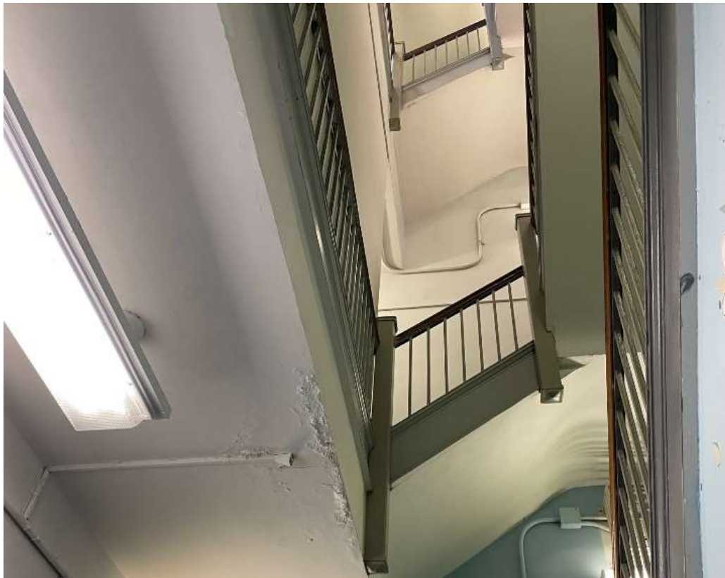
Photo A10 – View of stair #2, and damaged ceiling.
