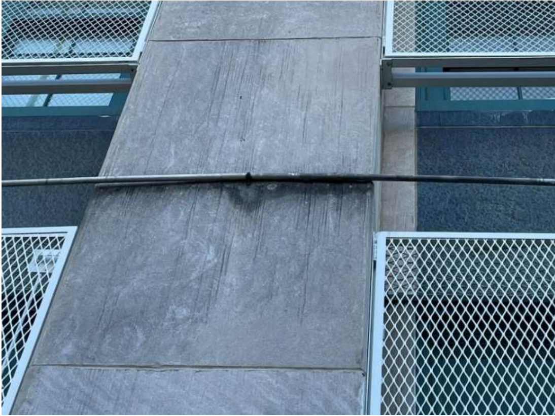
Photo M31 – Deteriorated mortar joints at all Facades.
