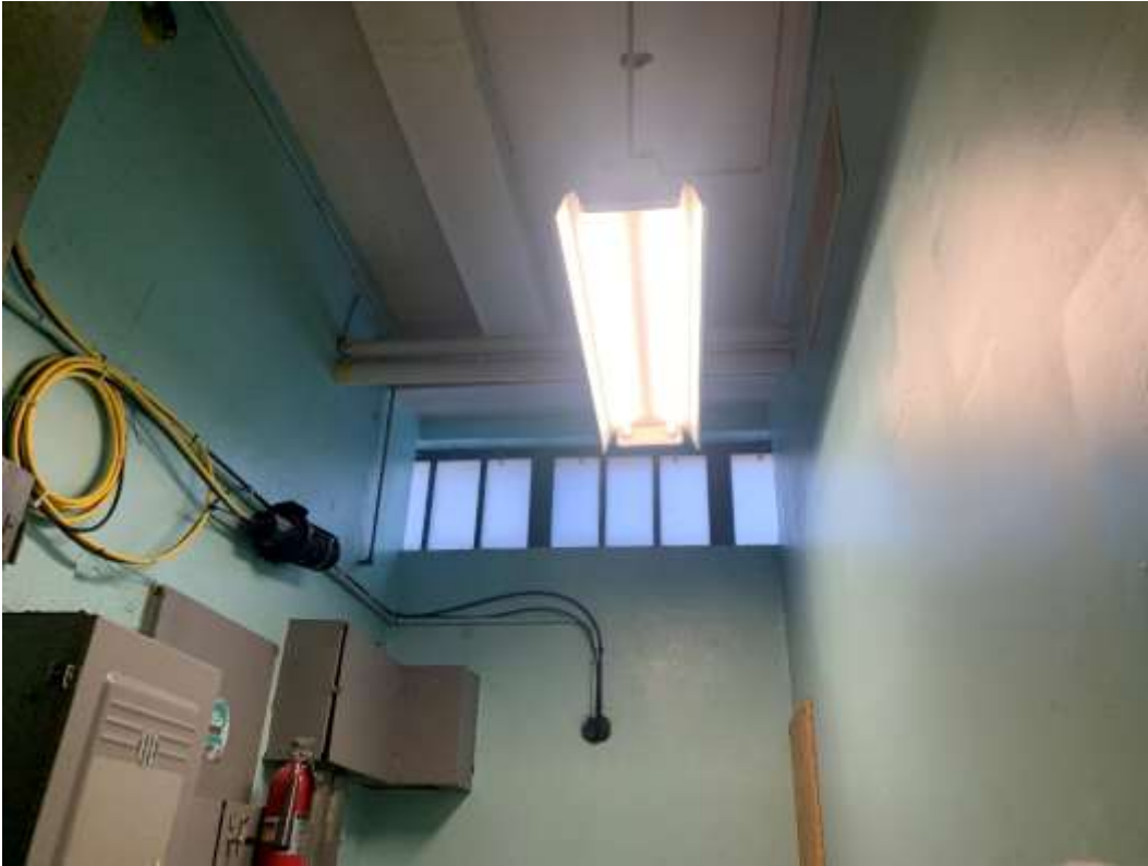
Photo A01 – View of electrical closet B2B.
