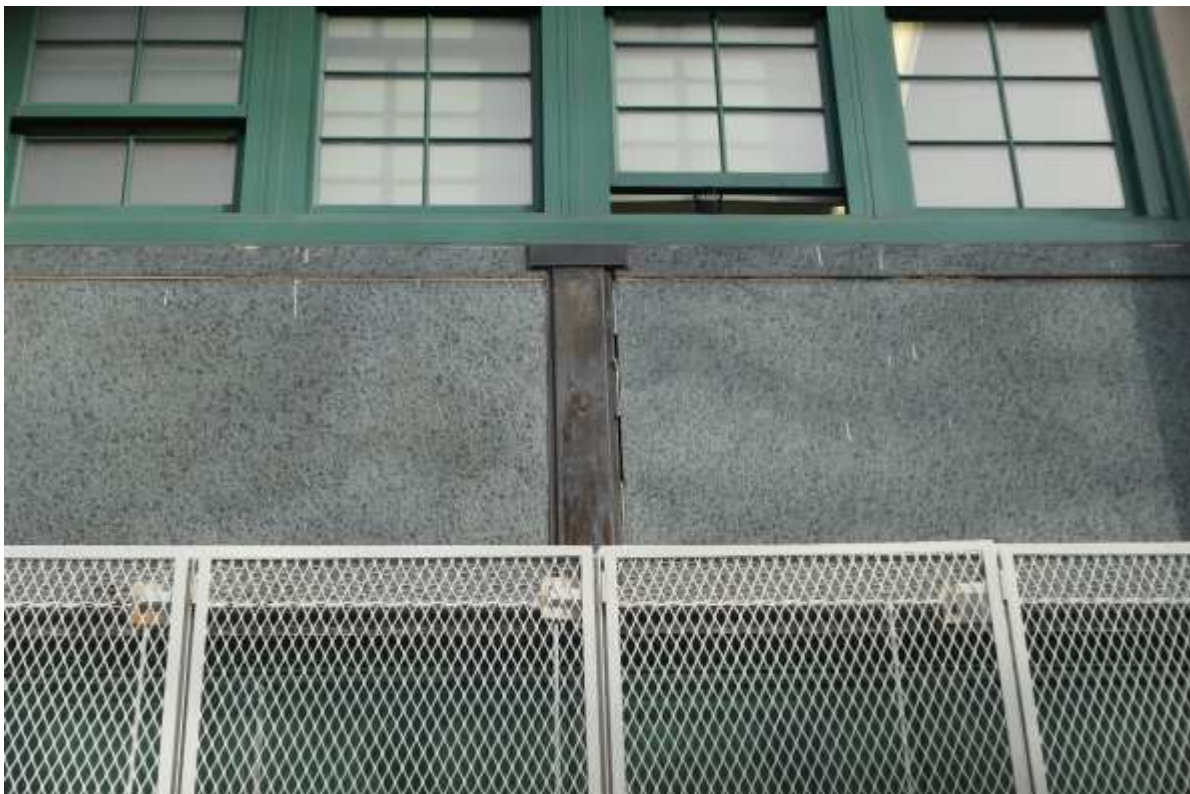
Photo M18 – Deteriorated mortar joints at granite panels.
