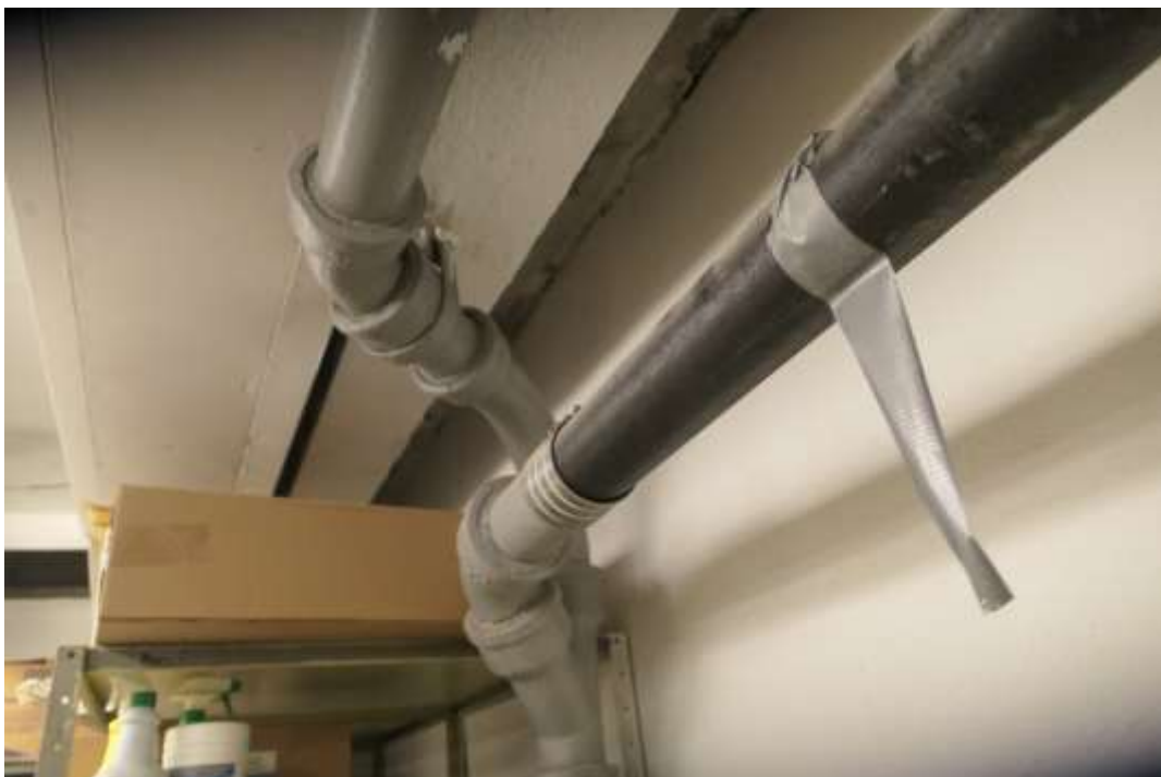
Photo A16 – Source of water infiltration is located at the ceiling line of Storage Room B4.
