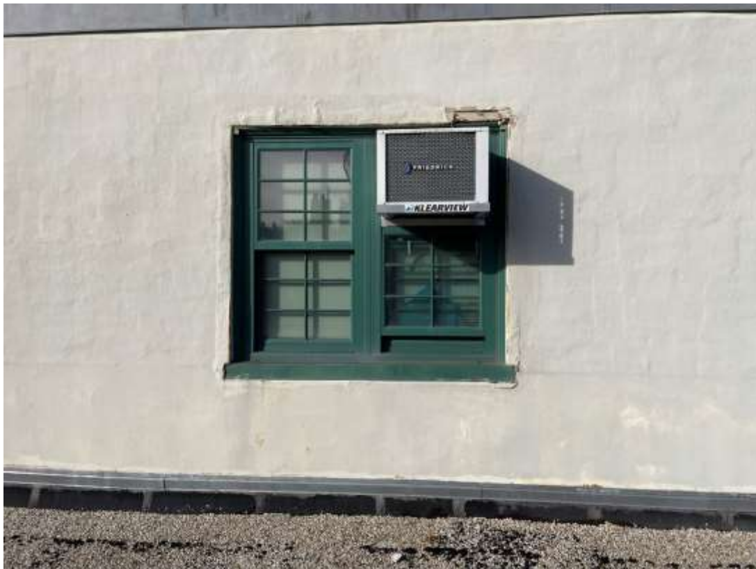
Photo M54 – Damaged stucco and missing stucco in windows perimeter indicates water infiltration – East Bulkhead Façade.
