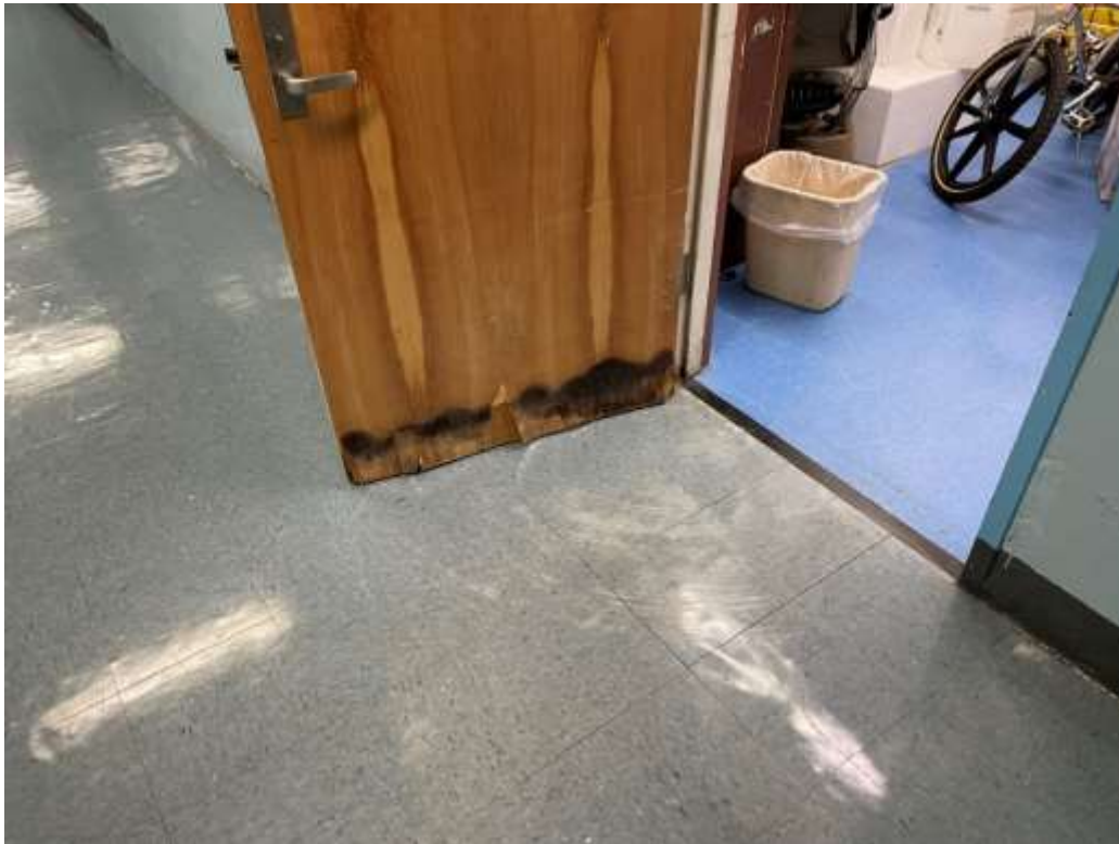
Photo A09 – Door water damage in Storage room B4.
