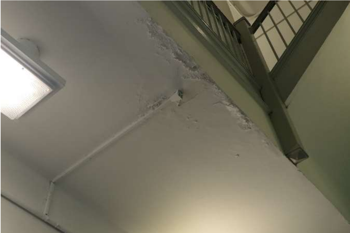
Photo A07– Deteriorated ceiling at basement stair #2.
