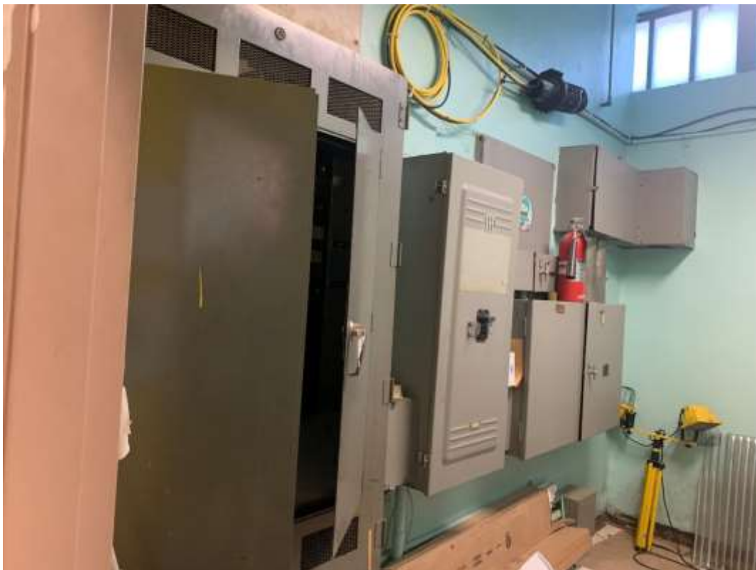
Photo A02 – View of electrical closet B2B.
