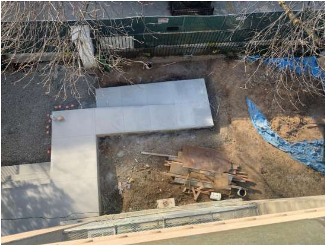
Photo S02 – View of existing ramp in construction at main entrance, taken from Roof.
