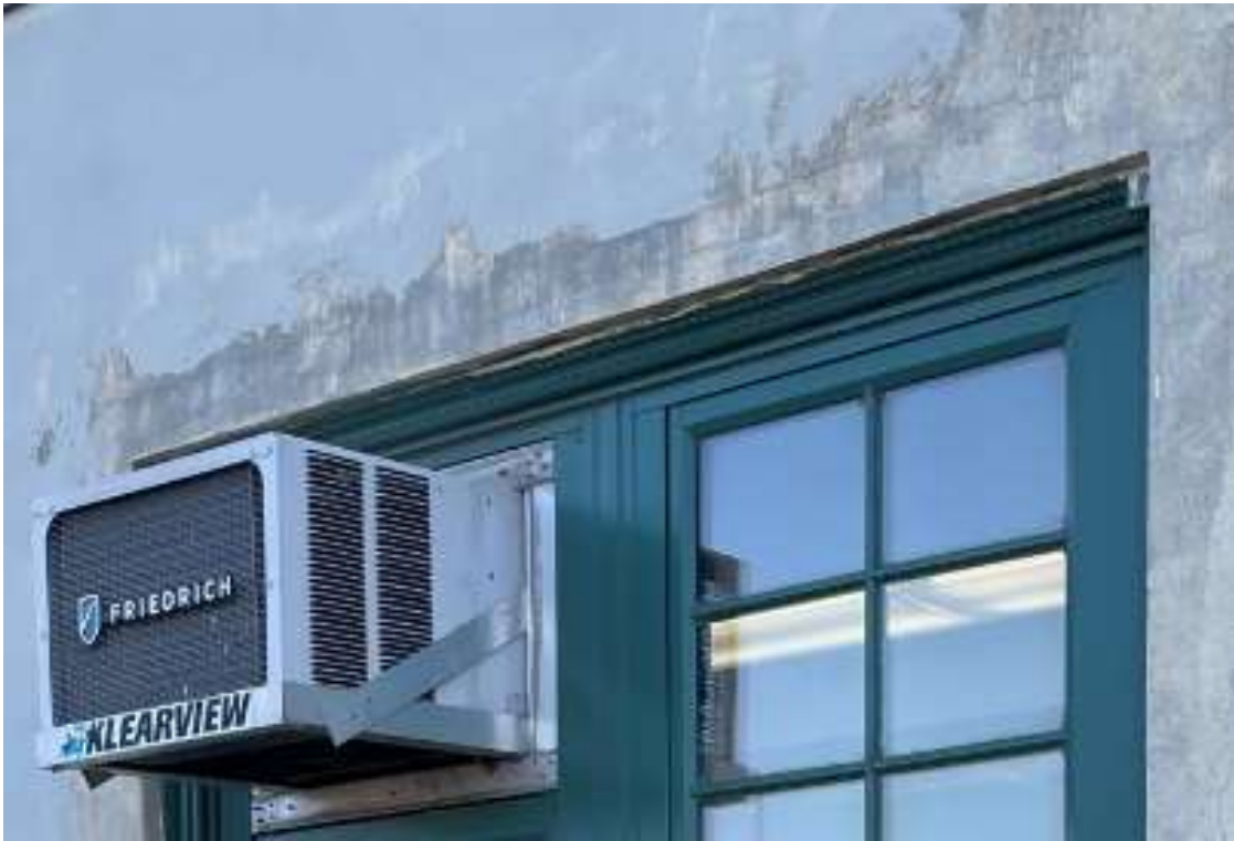
Photo M51 – Damaged stucco in windows perimeter indicates water infiltration – North Bulkhead Façade.
