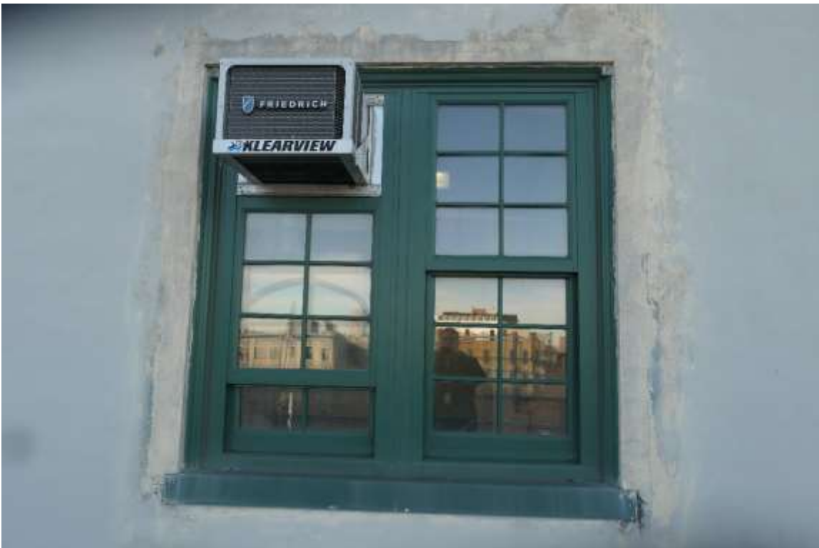
Photo M50 – Damaged stucco in windows perimeter indicates water infiltration – North Bulkhead Façade.
