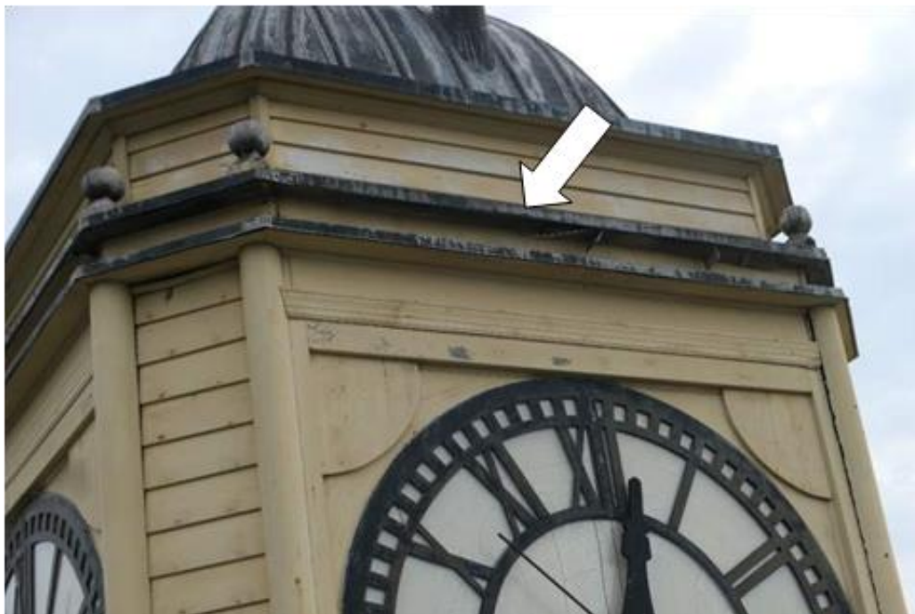
Photo 9 – Exterior view of ledges and flashing. Source of water penetration.
