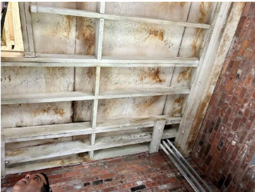
Photo 11 – View of framing and underside of plywood cupola flooring. Water staining and areas of rotted wood observed. This is consistent on all four faces. Trim and panel infill around clock faces is severely rotted.
