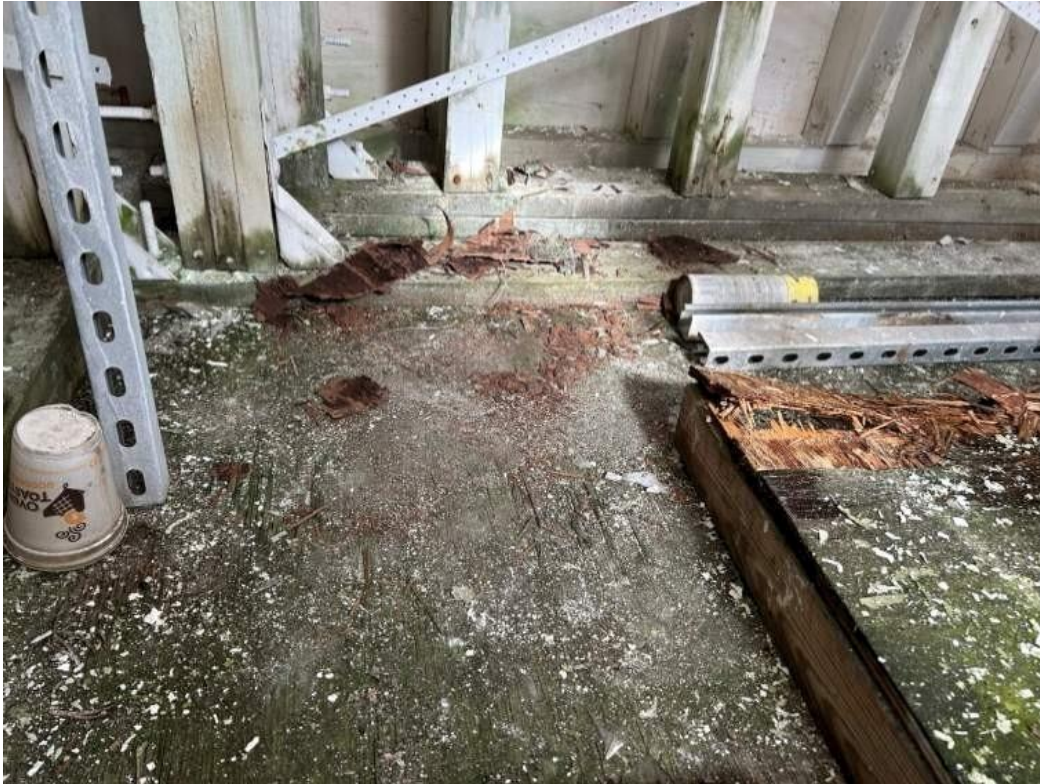
Photo 10 – Plywood flooring of cupola is rotted.
