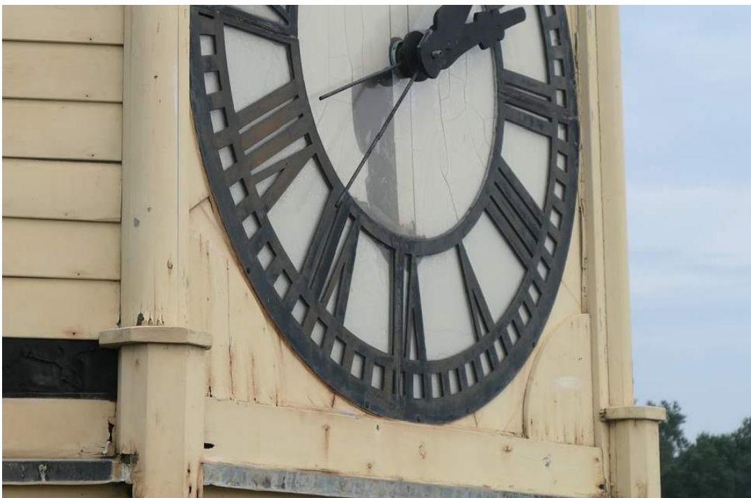
Photo 14 – Exterior metal dial, numerals and clock hands have a faded finish with some pitting noted. Refinish.
