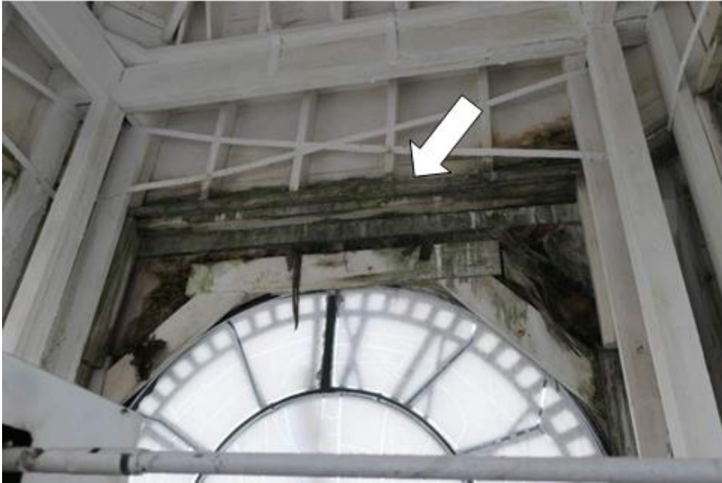
Photo 8 – Source of water penetration is two exterior ledges. This is consistent on all four faces. Trim and panel infill around clock faces is severely rotted.
