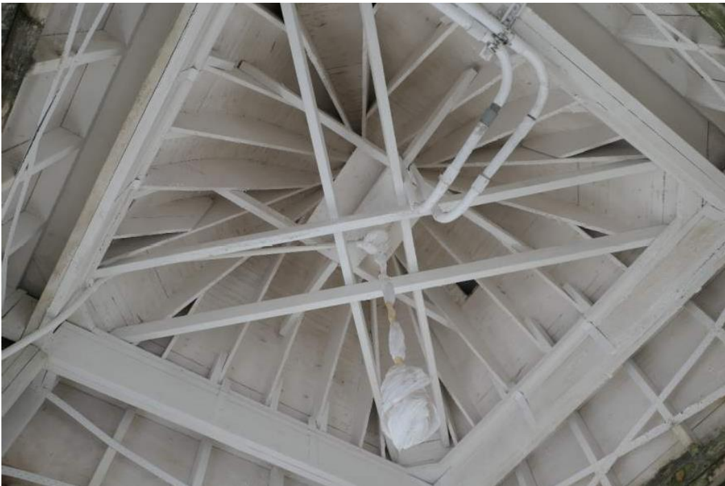
Photo 6 – Upper roof framing seen from the interior. No water staining or areas of rotted wood observed. No leaks from copper roofing. Light fixture is wrapped in plastic.
